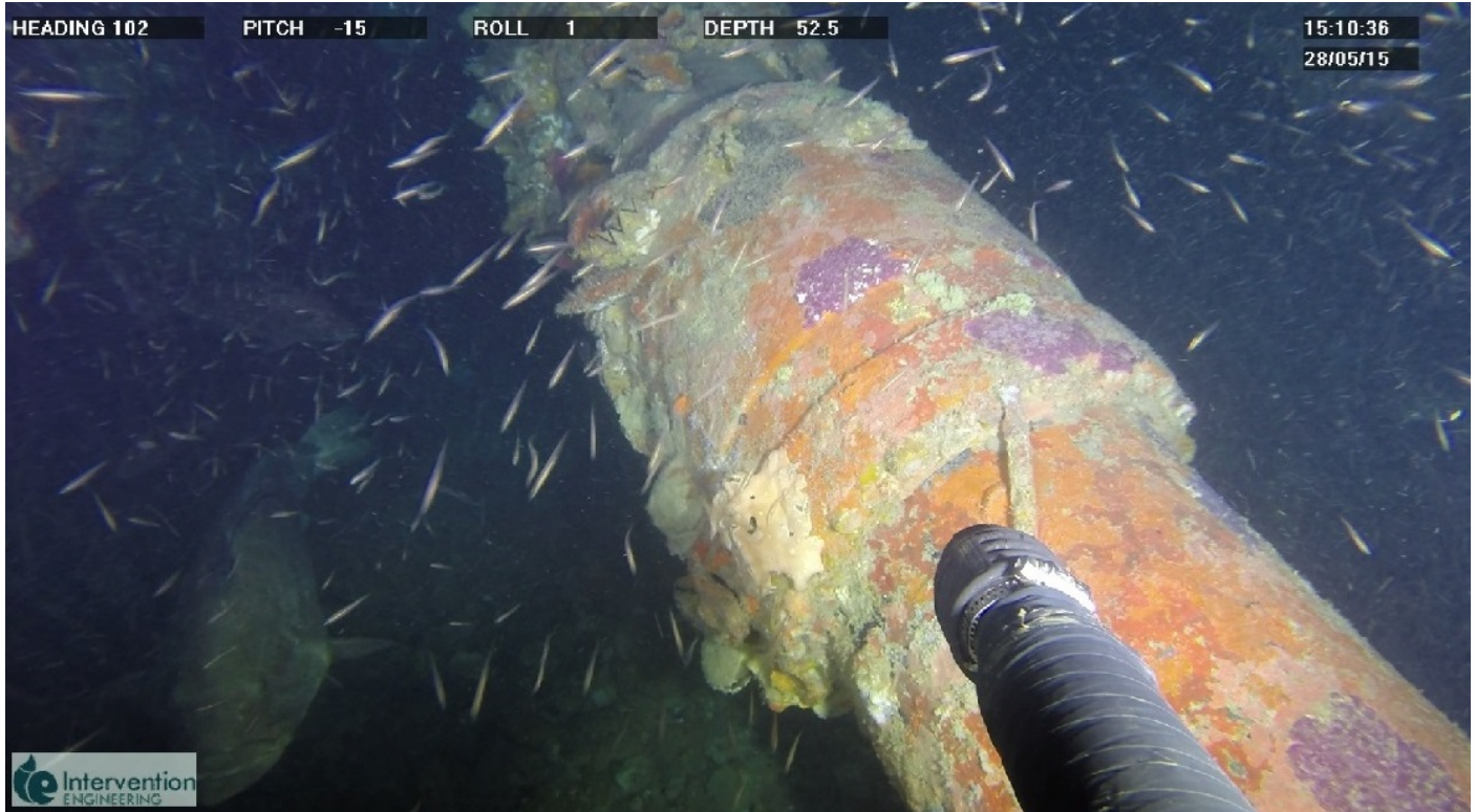
Before cleaning showing almost total coverage of soft growth
