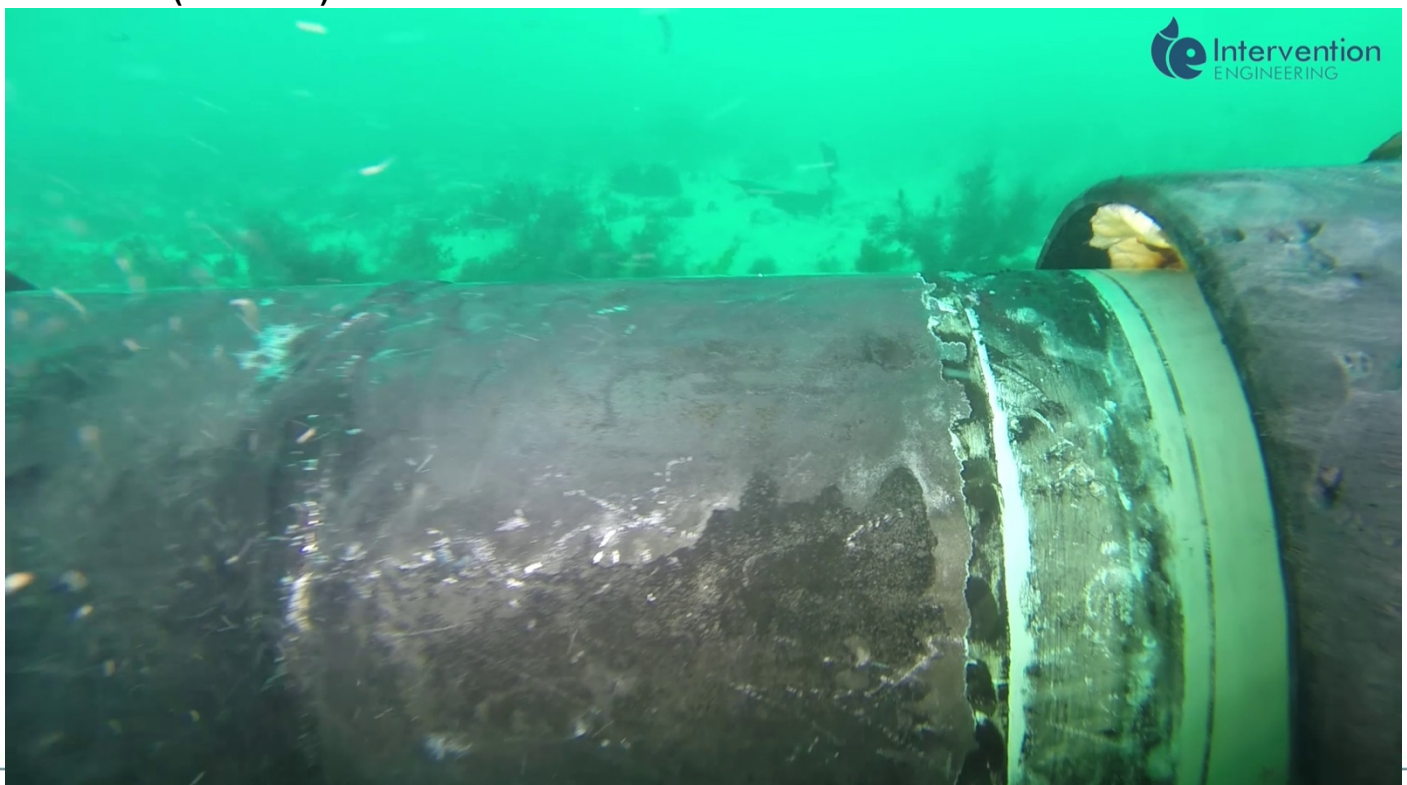
For this application we removed exterior wraps to expose the joint for UT scanning
