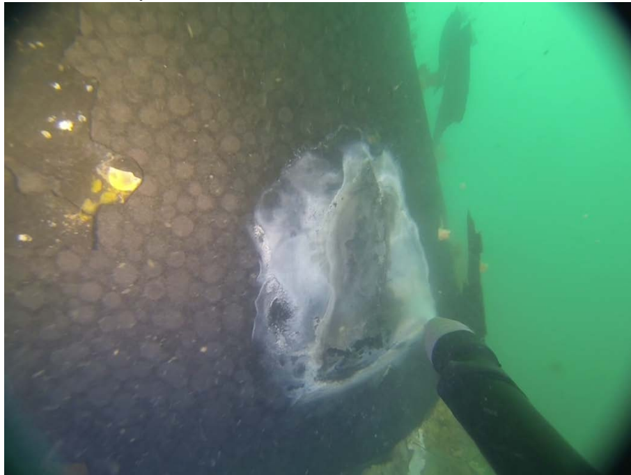
Cleaning a pile – poor coating adhesion and areas of corrosion evident
